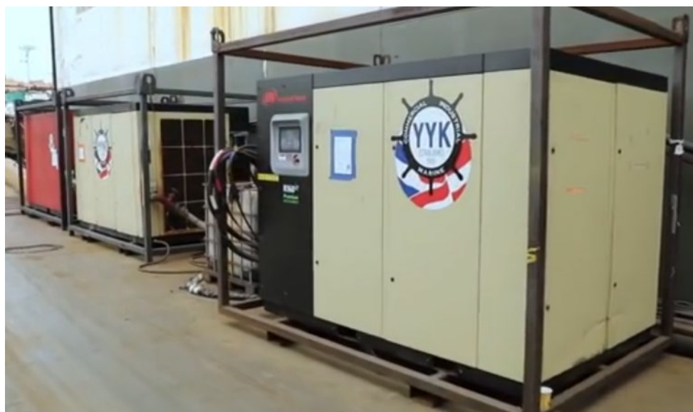
Figure 3-3. Electric Compressors at NASSCO
