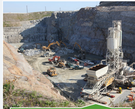
Concrete Batch Plants
