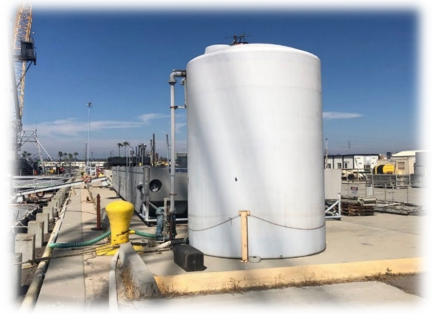
Storm Water Diversion
