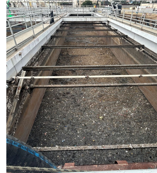
PST 5 Sediment Buildup after 2 months in operation
