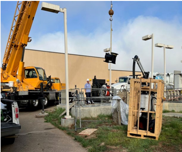
All 4 Pumps replaced in the last year post TS Hilary
